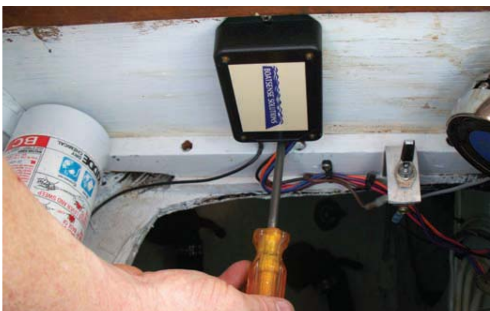
PS testers mounted the Boatsense monitor beneath the helm and near the high-water alarm of a Union 36 test boat. The install took about 1½ hours.
